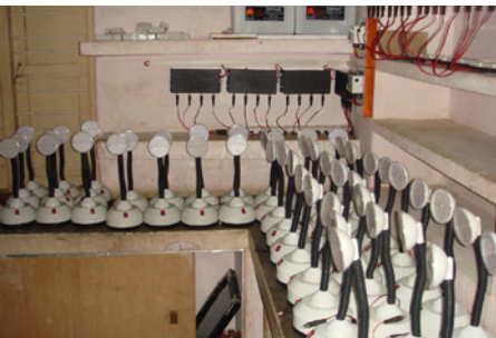
Solar lamps and charging station
