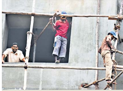
Safety regulations are violated with impunity at BBMP headquarters, where labourers working on a new building face danger at every step —Anantha Subramanyam K
